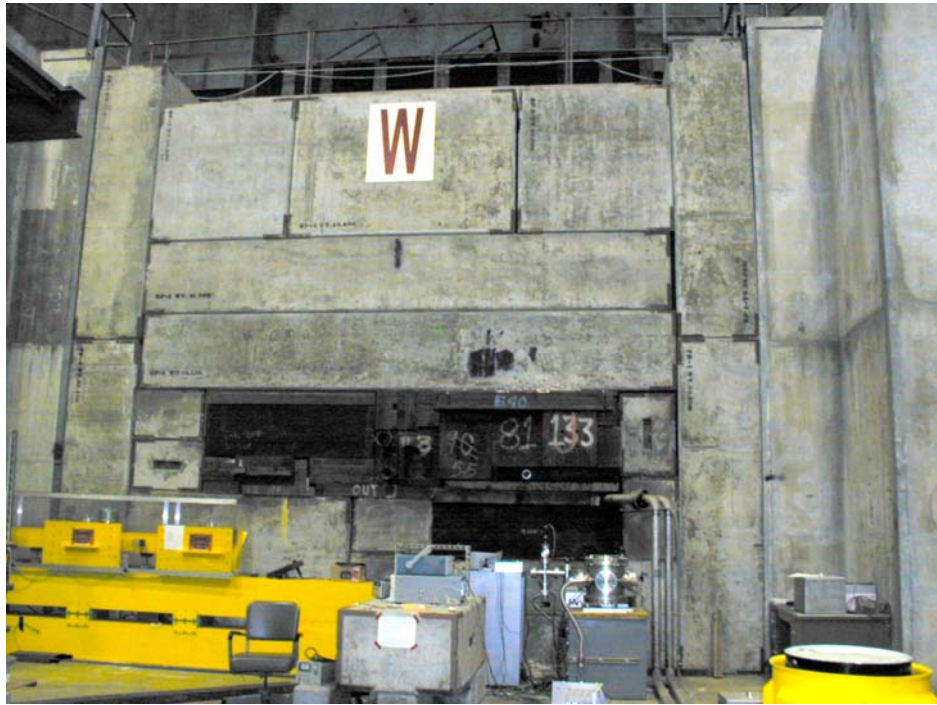
Picture of concrete shielding block stacked without seismic ties.
