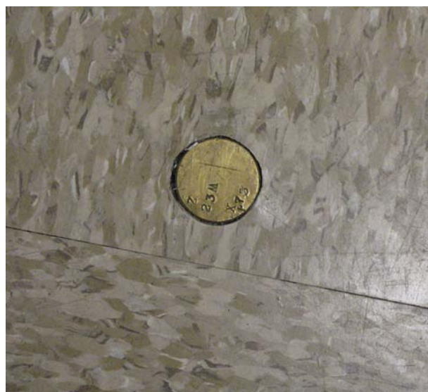
A Brass Plug Installed in Floor
