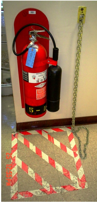
Figure 1 Example of Floor Taping for a Fire Extinguisher
