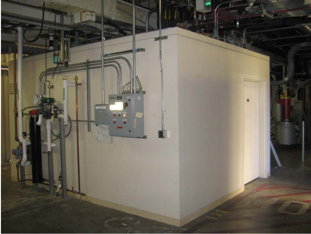
Figure 5-21. Enclosure for precision LCLS equipment in the Klystron Gallery. A structure similar to this will be constructed near klystron station 20-6. Data acquisition systems or other electronic equipment that must be near the beam could be set up here, directly above the experiment area in the linac tunnel 25 feet below.
