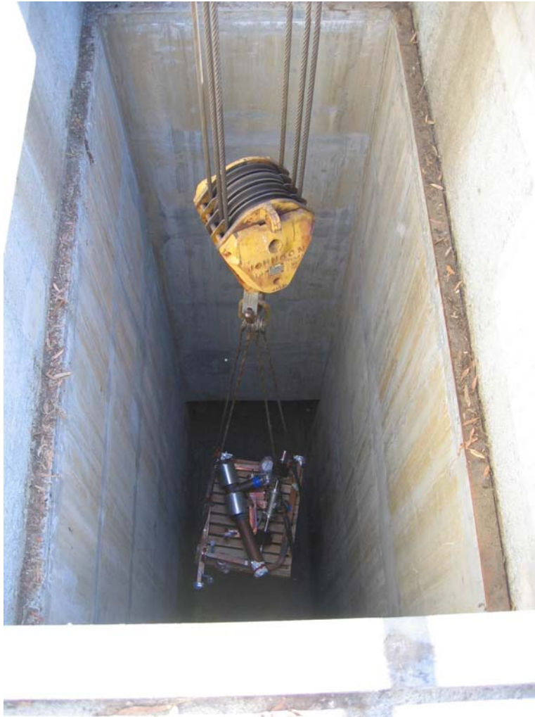
Figure 5-18. Pallet of equipment being raised through the equipment shaft in Sector 19 near the ASF focusing system. Identical shafts exist at five-sector intervals along the linac.
