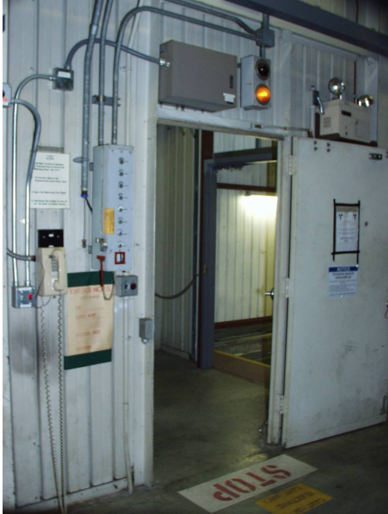
Figure 5-19. Personnel access door leading from the Klystron Gallery to the linac tunnel in Sector 24. The stairway and PPS controls will be copied in Sector 19.
