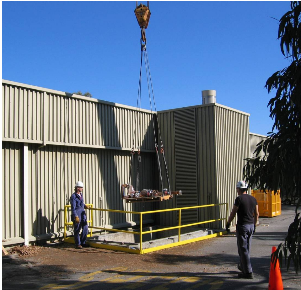
Figure 5-17. Equipment access shaft in Sector 19 along the south road of the Klystron Gallery. A pallet of equipment is being lifted out of the shaft with a portable crane. Identical access shafts exist at five-sector intervals along the Klystron Gallery.
