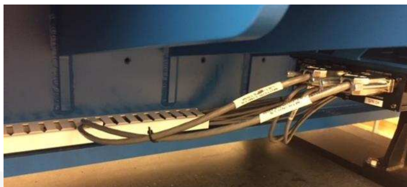
Figure 115: Limit Switch Interface box. Wall Side.
