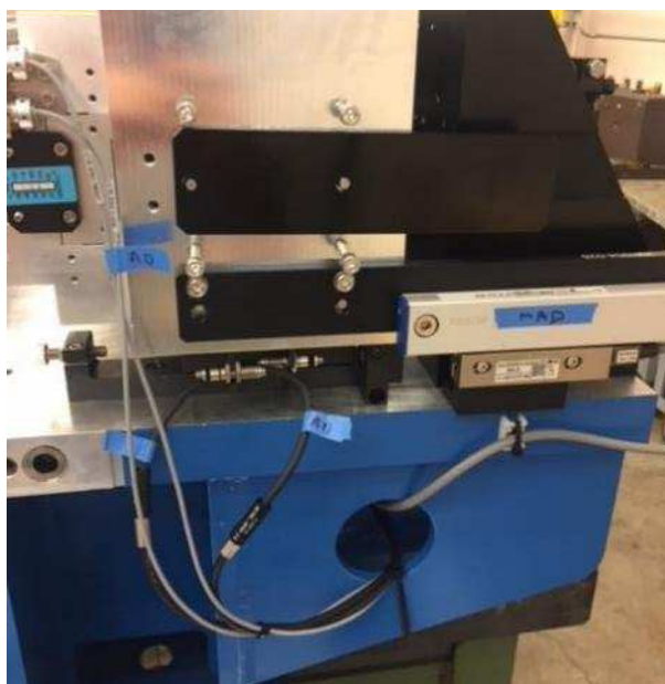
Figure 117: Downstream, Aisle vacuum chamber switches, hardstop switches, half-gap encoder wiring
