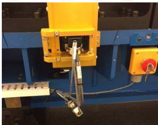
Figure 113: Motor and E-stop cables into Panduit. Aisle Side.
