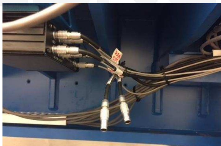
Figure 116: Limit switch interface box. Wall Side. Note 2 connectors are disconnected. These are the dummy vacuum chamber switch cables. The vacuum switch and dummy vacuum switch share their input connector.
