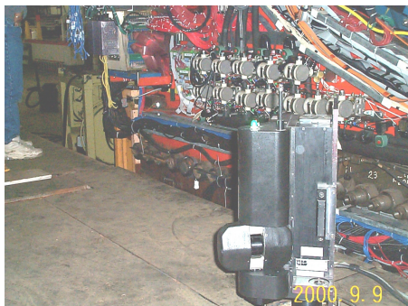
Figure 21 – SMX 3000 on west side
