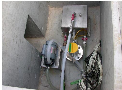
Fig.6 Inside of the HLS pit
