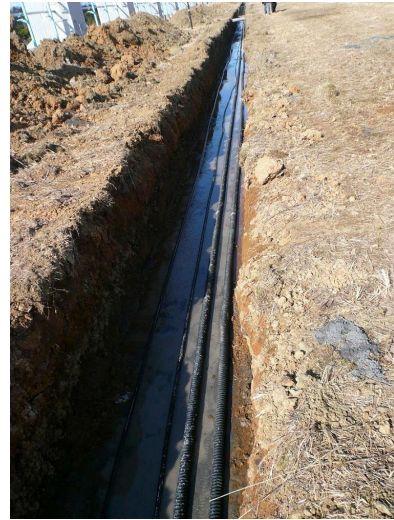
Fig.4 Communication pipes connecting HLS sensors are laid in same level of -1m.
