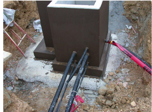
Fig.5 Communication pipes, the lowers are for water and uppers are for air and cables.
