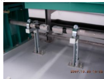
Fig.8 picture of pipe and bolsters
