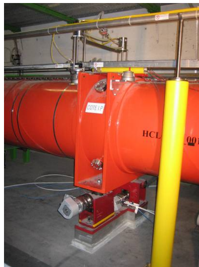
Fig. 2: Sensors and motors installed on a low beta quadrupole
