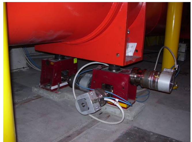
Fig. 4: Motor assemblies plugged on jacks
