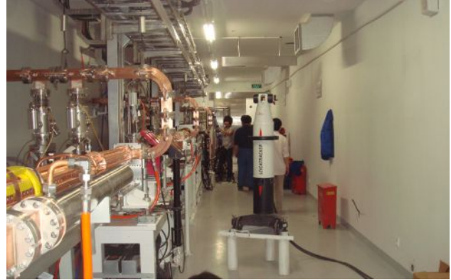
Figure.12: Tunnel installation of linac
