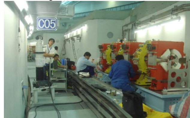
Figure.13: Tunnel installation of storage ring
