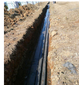
Communicating pipes connecting HLS sensors
