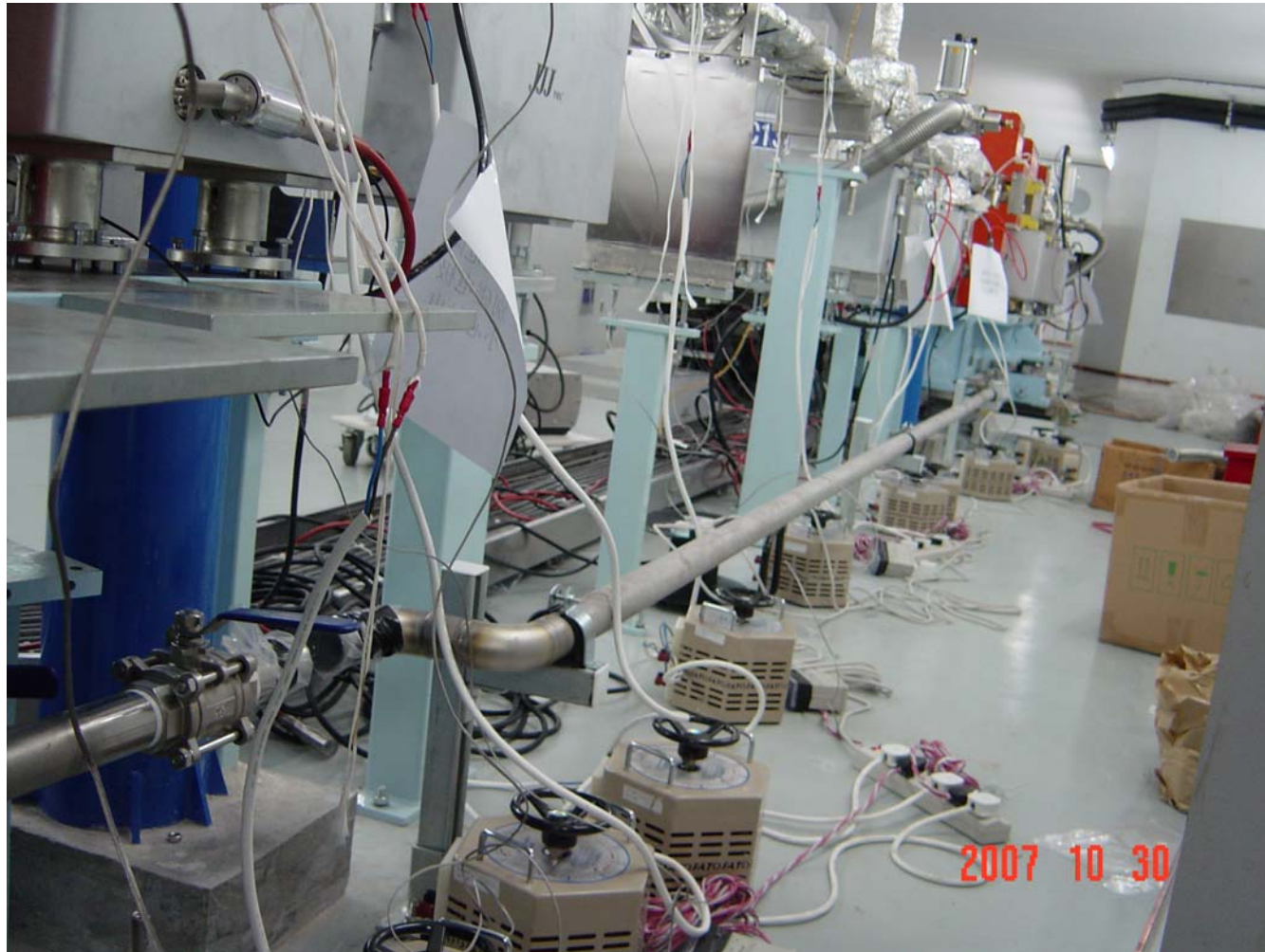
Water pipe in SR
