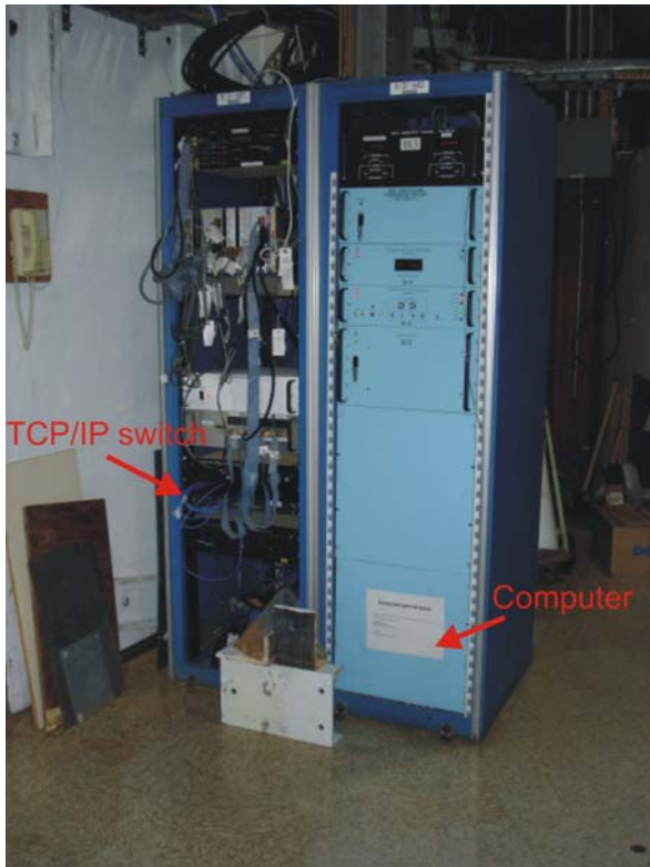
Figure 6: Electronic rack B160-131 with HLS computer and TCP/IP switch
