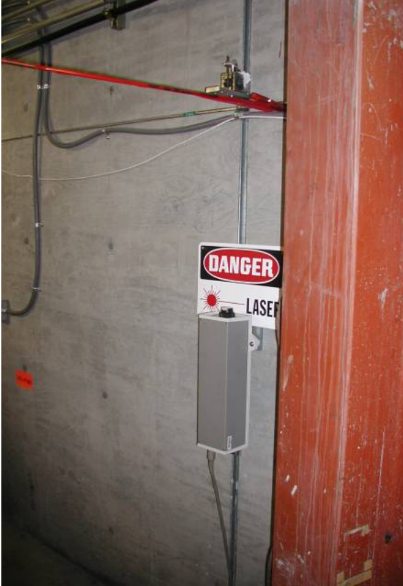
Figure 5: Mount of the laser head and the interferometer on the wall
