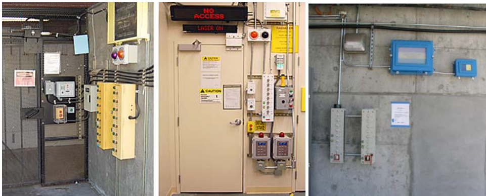
Figure 7-1 Three Examples of Personnel Protection Systems at SLAC
