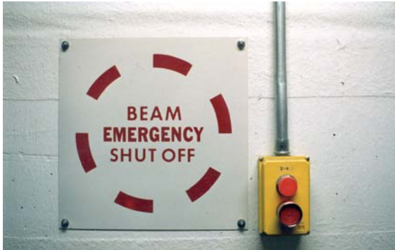
Figure 8-2 EMERGENCY OFF Button
